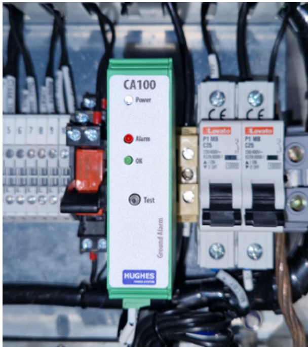
Installation in the motor drive cabinet
